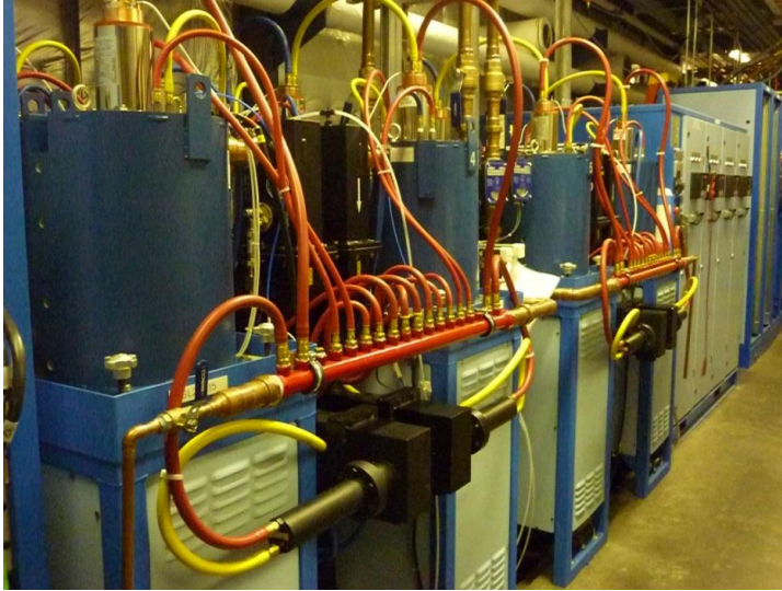
Figure 3: 12 GeV Klystrons. One per Cavity
