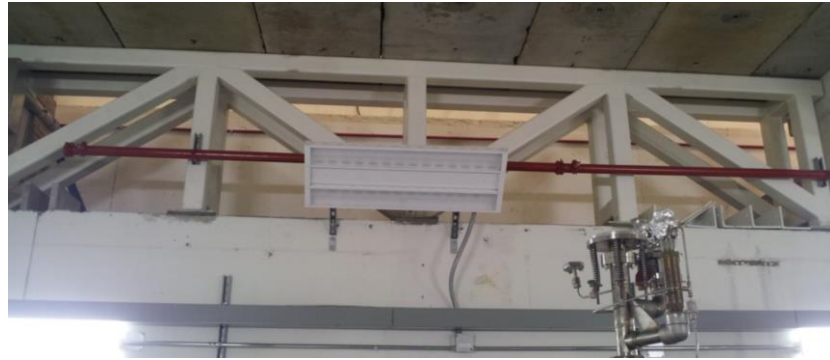
Figure 15: (top) Shielded elevated-roof section of Cave 2, which will be used for experimental targets, including cryogenic targets. (bottom) 5.6 m 2 Vent area beneath the elevated roof section of Cave2, for lighter than air cryogenic gases to escape.
