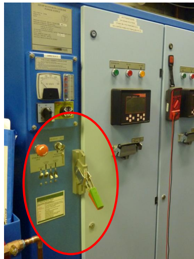
Figure 6: Klystron Power Supply with Knife Switch Highlighted
