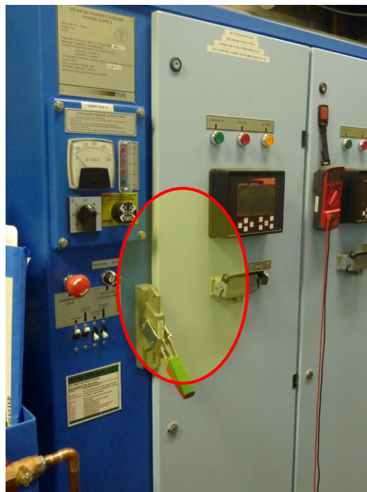
Figure 4: Location of HV Power Supply Knife Switch
