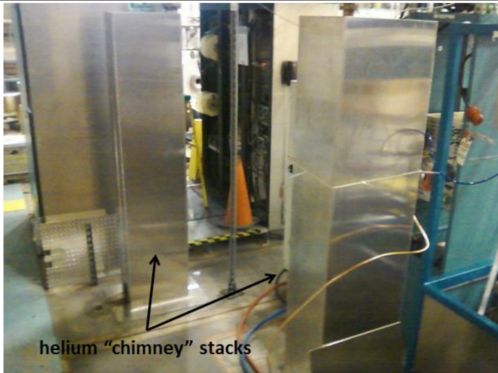
Figure 14. Two helium “chimney” stacks attached to rectangular penetrations in the ceiling of Cave 1. If helium gas is released inside the UITF enclosure, these chimneys will direct helium gas above the heads of staff members working near the electronics racks above Cave 1. Before energizing the QCM with high power RF energy, sandbags will be positioned at the base of each “chimney”.
