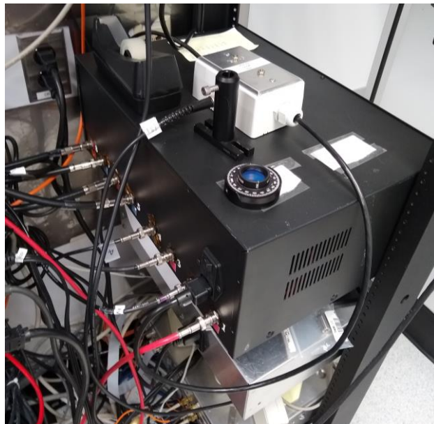
Figure 6: RTP Pockels cell HV supply used at CEBAF laser table.
