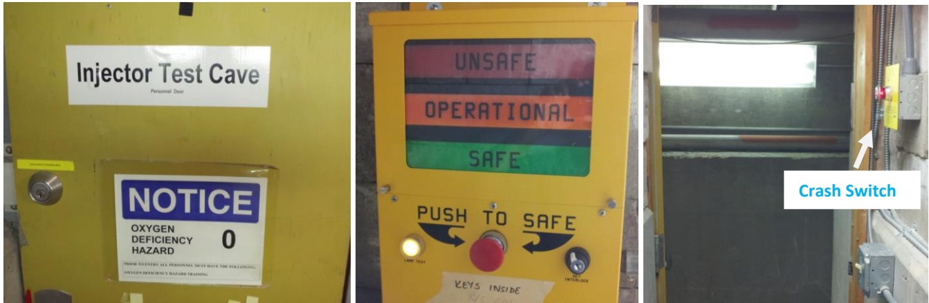
Figure 14 (Left) Exit door into high bay from Cave 1 near the electron gun (Middle) Run/Safe Box (Right) Crash Switch for exit. Run/Safe Boxes and Crash switches are at both the entrance/exit ways
