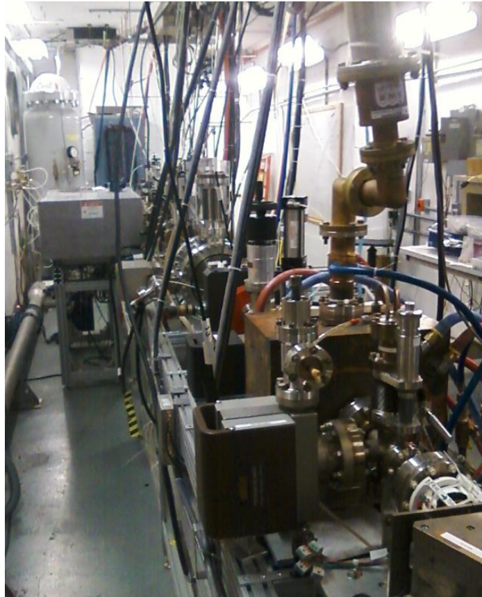
Figure 7: Photograph of the buncher installed on the keV beamline at UITF, looking toward the photogun.
