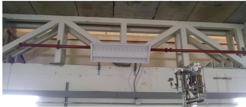
Figure 18: (top) Shielded elevated-roof section of Cave 2, which will be used for experimental targets, including cryogenic targets. (bottom) 5.6 m 2 Vent area beneath the elevated roof section of Cave 2, for lighter than air cryogenic gases to escape.
