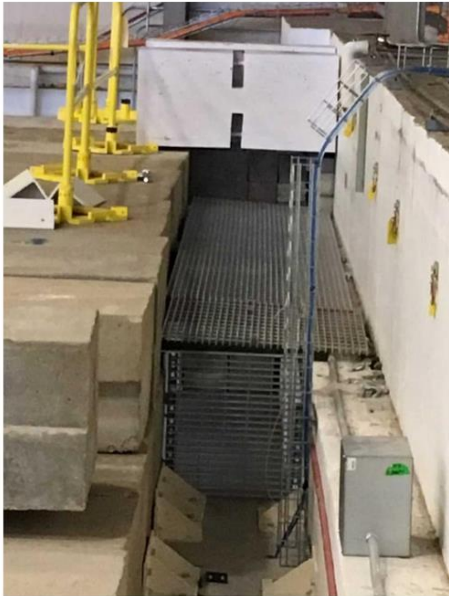
Figure 11: the grating at the Cave2 helium vent that prevents entry into the UTF enclosure. Attached signage designates the grating as UTF credited control but is not shown in this photograph.
