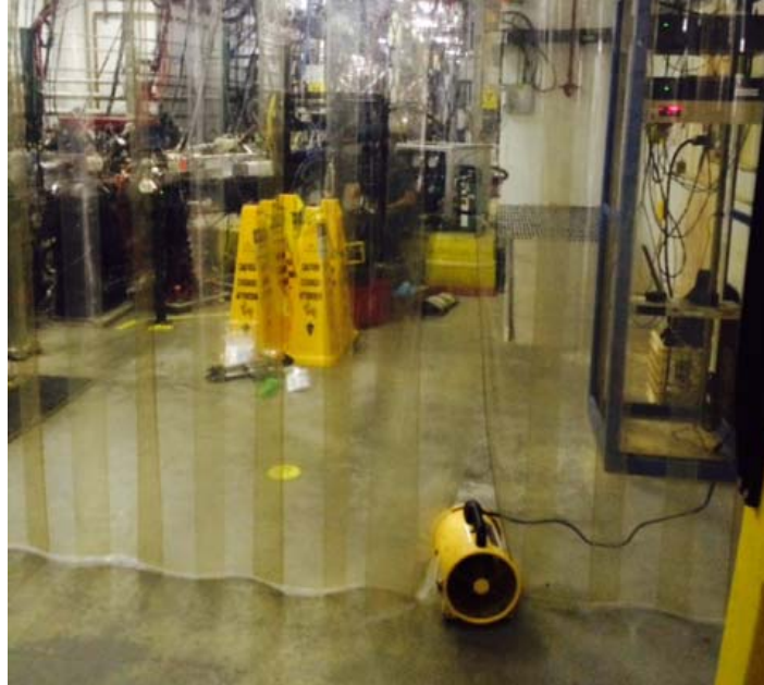
Blower positioned in tunnel to promote mixing during nitrous oxide venting.
