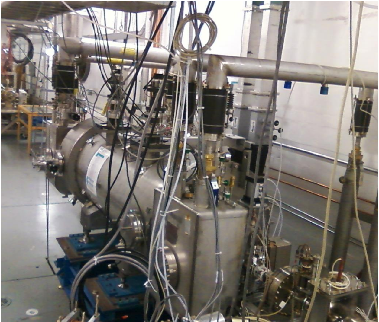
Figure 17, top and bottom: The QCM in position at Cave1 of the UITF, with u-tubes “stabbed” and waveguides connected.
