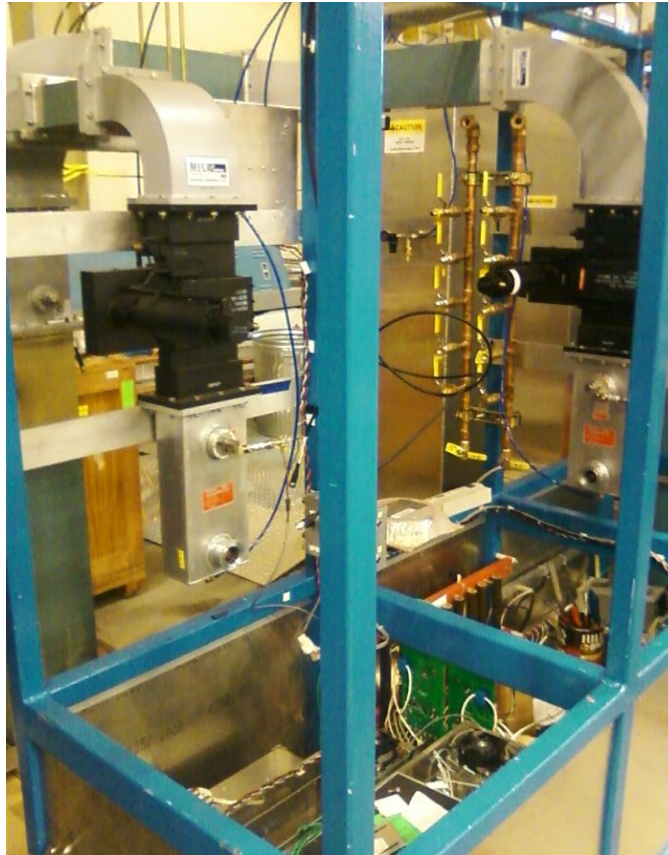
Figure 11, the UITF klystron racks under construction. Photo will be updated when construction is complete.
