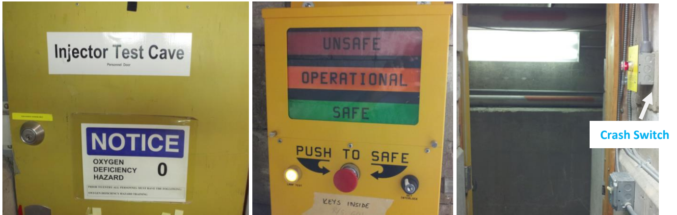
Figure 9 (Left) Exit door into high bay from Cave1 near the electron gun (Middle) Run/Safe Box (Right) Crash Switch for exit. Run/Safe Boxes and Crash switches are at both the entrance/exit ways
