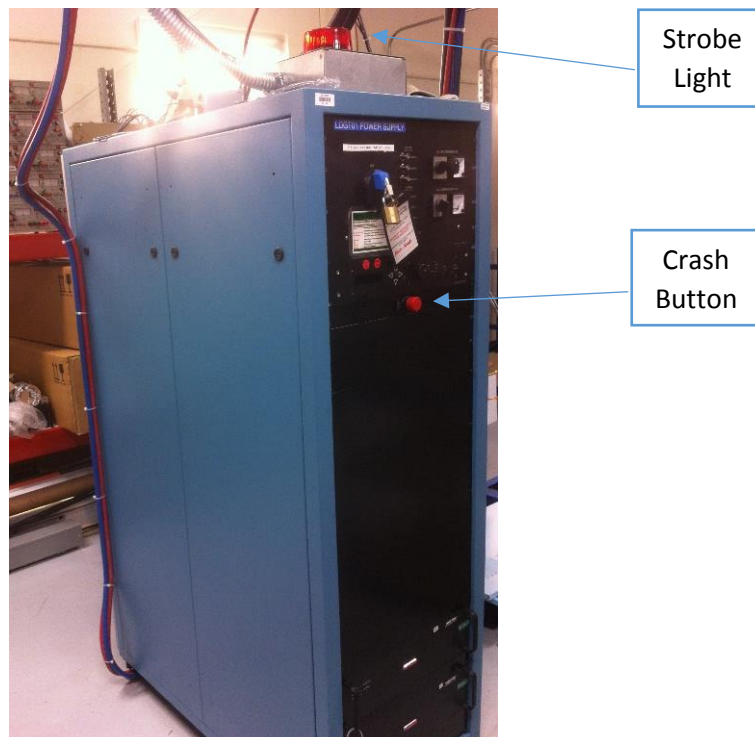
Figure 2: Magnet power supply at the GTS mezzanine. There is a crash button on the front panel.
