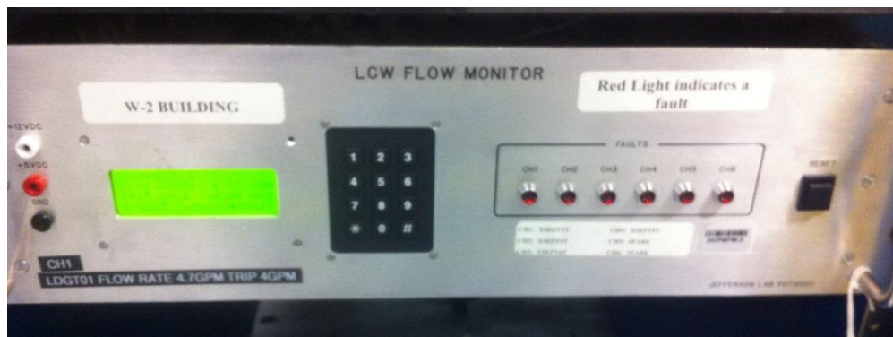
Figure 4: Cathode magnet LCW flow rate monitor chassis at the GTS mezzanine.
