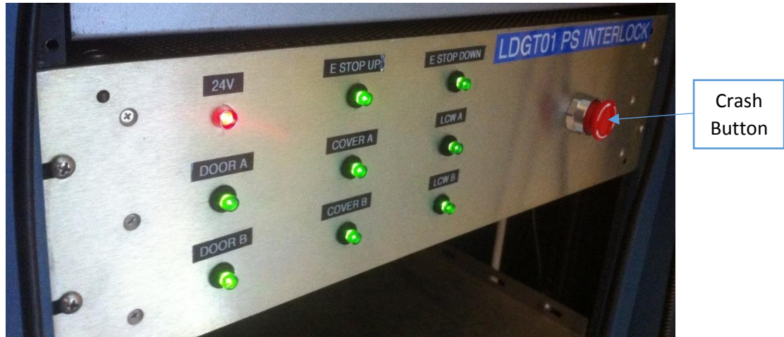
Figure 5: Cathode magnet power supply interlock box in the GTS control room.
