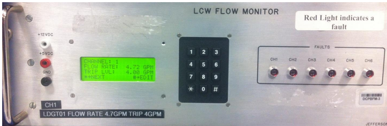
Figure 4: Cathode magnet LCW flow rate monitor chassis at the GTS mezzanine in Rack GL01B05. The status of this interlock is displayed in the control screen under “Solenoid LCW”.
