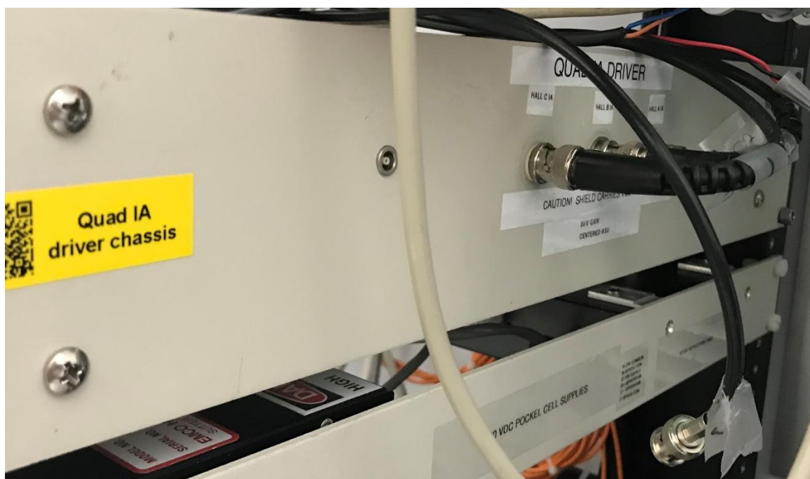
Figure 2: IA system HV supply and switch.
