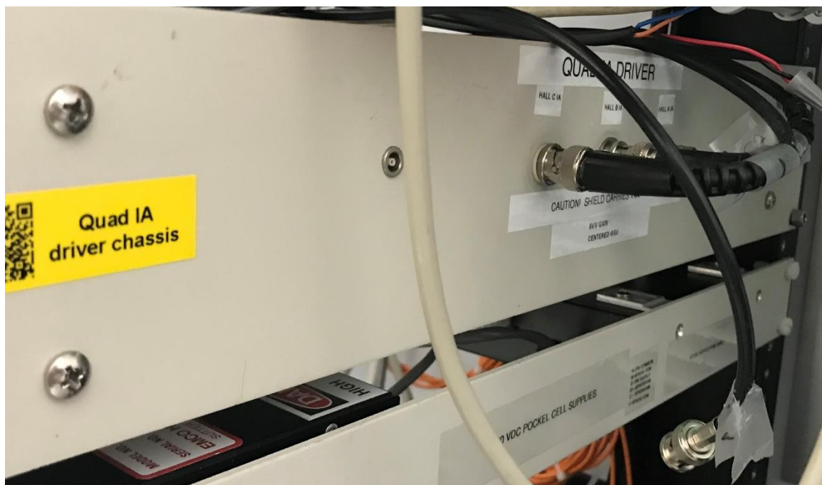
Figure 2: IA system HV supply and switch.
