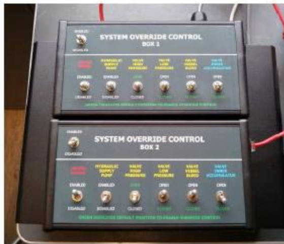
Figure 6: System Override Box
