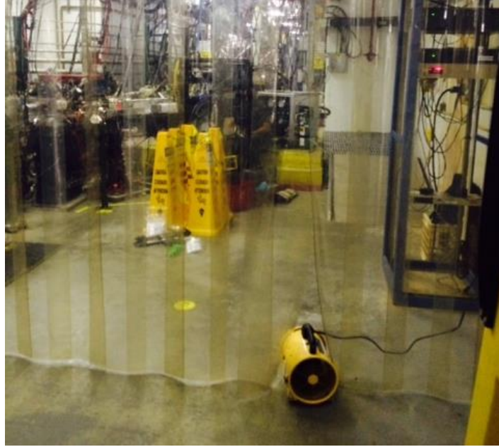
Blower positioned in tunnel to promote mixing air during nitrous oxide purging.
