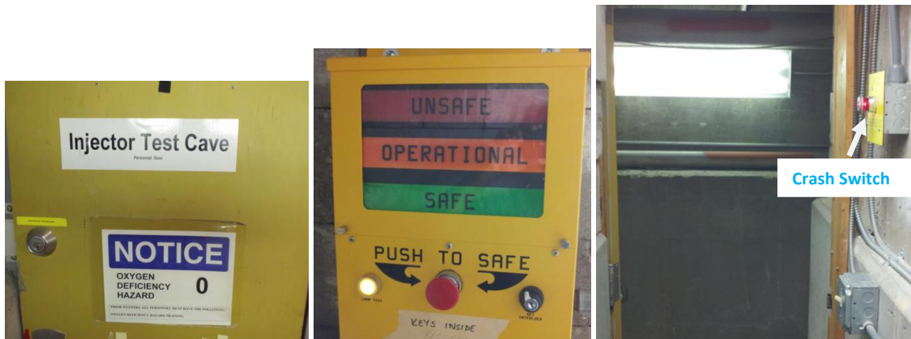
Figure 7 (Left) Exit into high bay from Cave 1 near the electron gun (Middle) Run/Safe Box (Right) Crash Switch for exit Run/Safe Boxes and Crash switches are at both the entrance/exit ways
