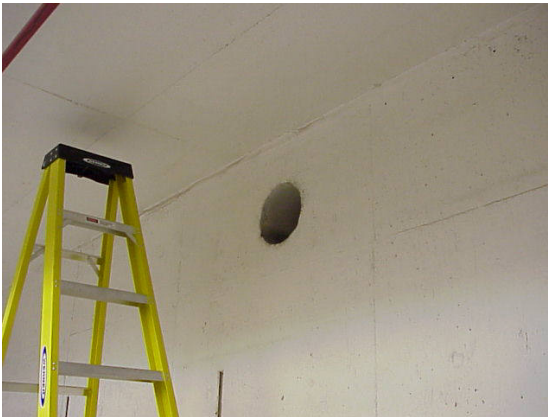
2 nd Floor Open Waveguide Vent
