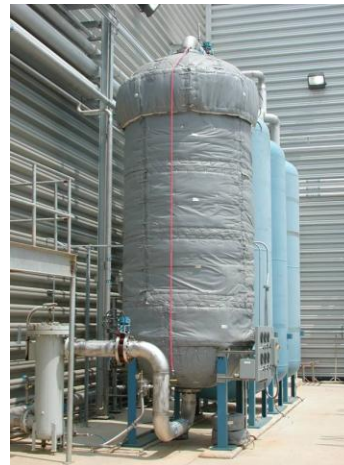
Oil Removal System
