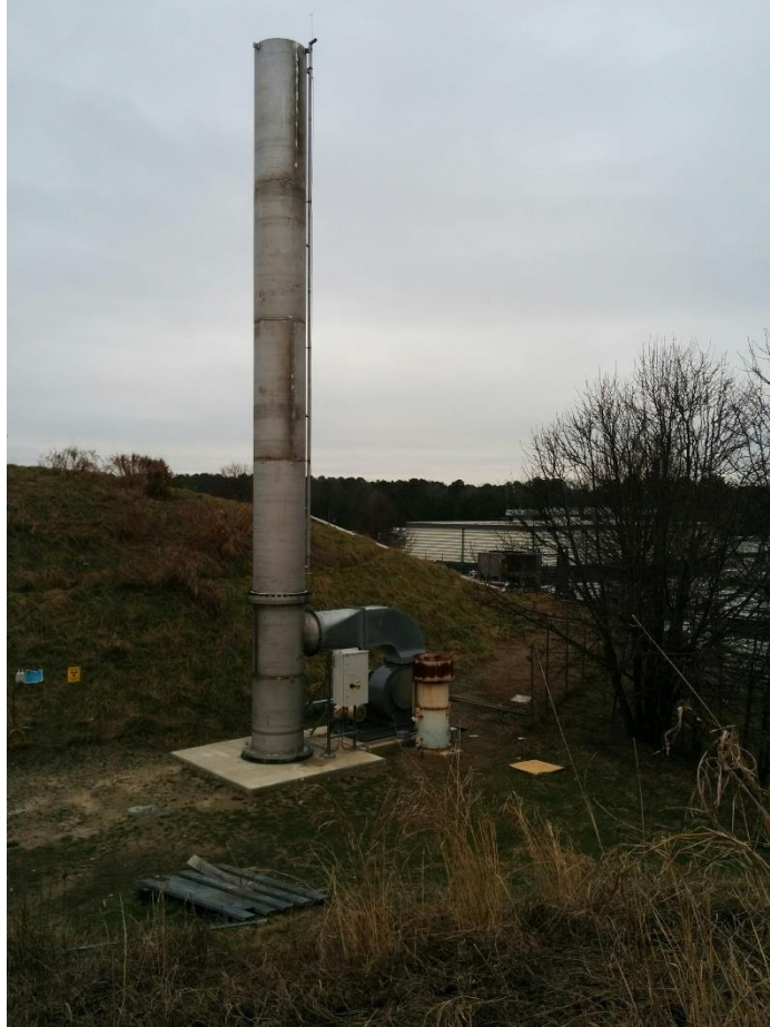
Figure 5: Tritium stack and blower located on the Hall A dome.
