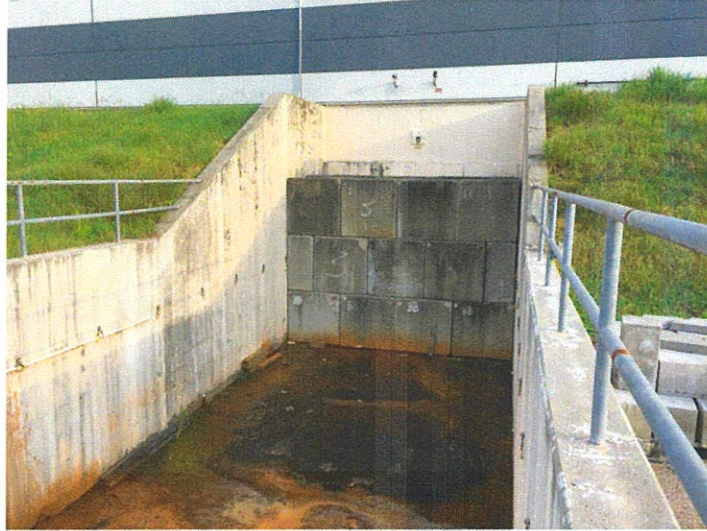
Figure 1: LERF truck entrance with concrete shielding in place
